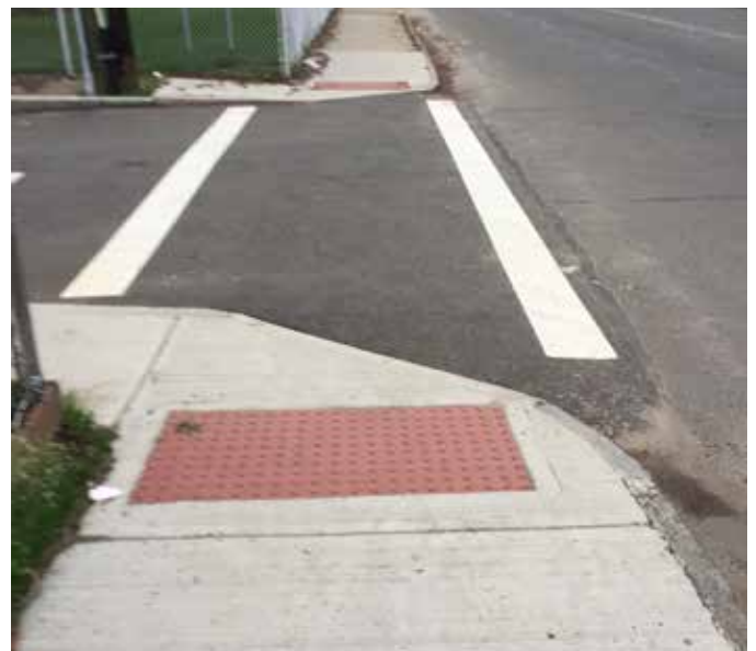
Some neighborhood sidewalks have been upgraded with new concrete and ADA-compliant curb ramps. Investments such as these need to occur throughout Old Hill.
