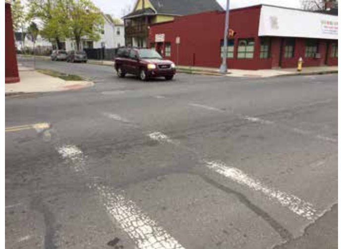
Existing crosswalks need to be repainted with enhanced pavement markings, such as a ladder or continental crosswalk design
