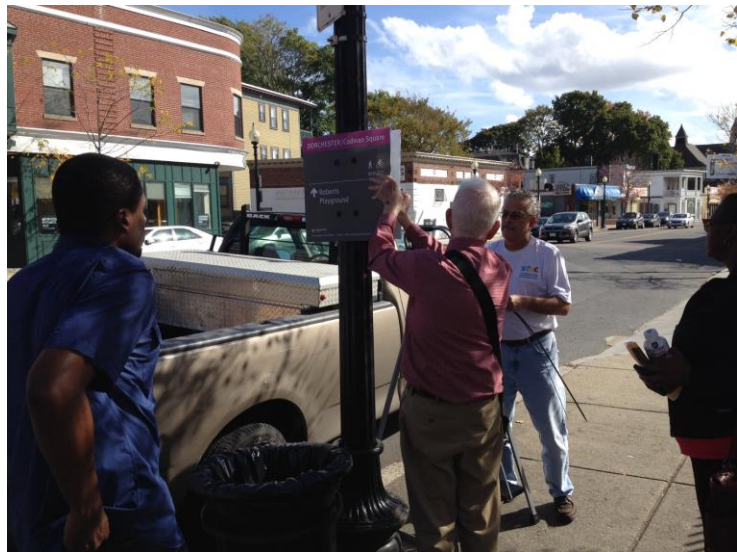
WalkBoston’s senior project manager Bob Sloane installs a wayfinding sign in Codman Square.
